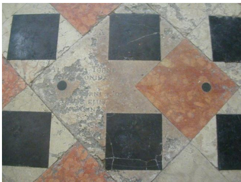
Figure 13: Example of Cracks
