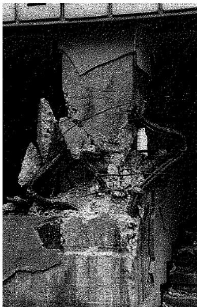
Figure 30: Confinement Failure of a Column (Paulay and Priestley 1992, 4)
