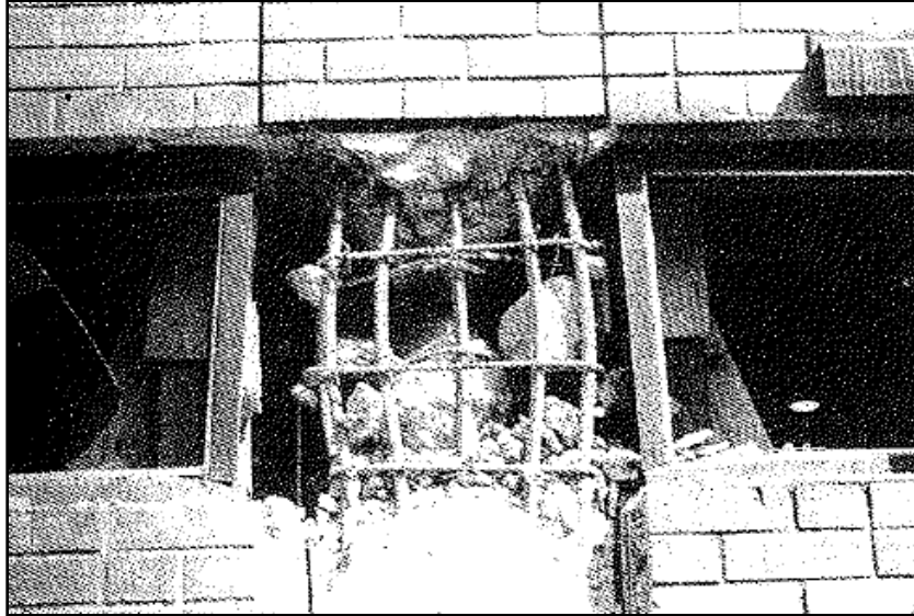
Figure 29: Confinement Failure of Column (Paulay and Priestley 1992, 5)
