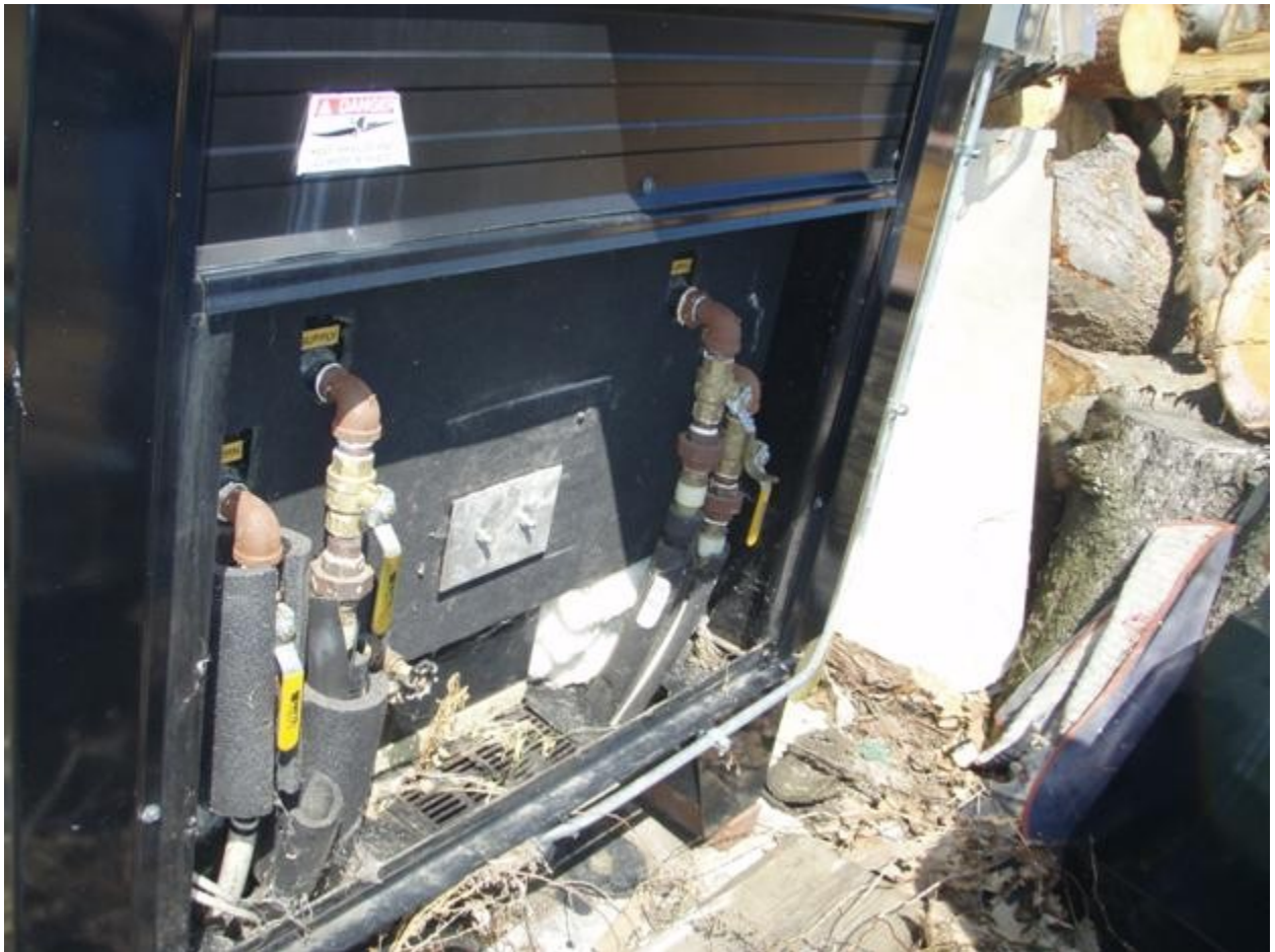
Figure 30: Pipe Attachments on Farmer E's Wood Boiler
