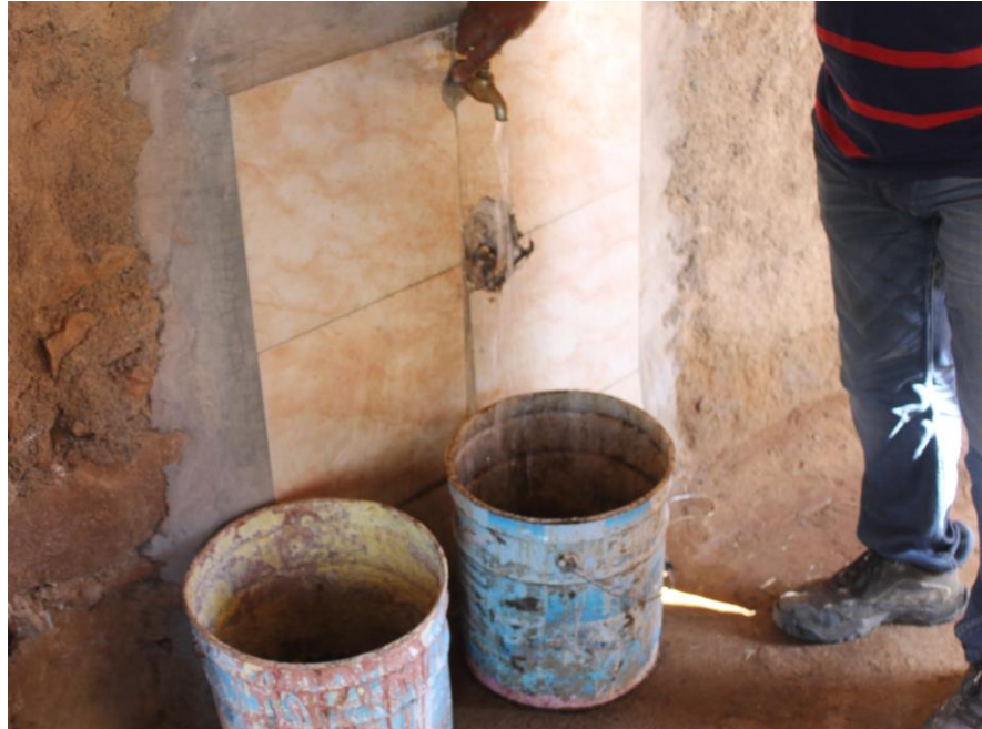
Figure 18: Water tap in one of the households
